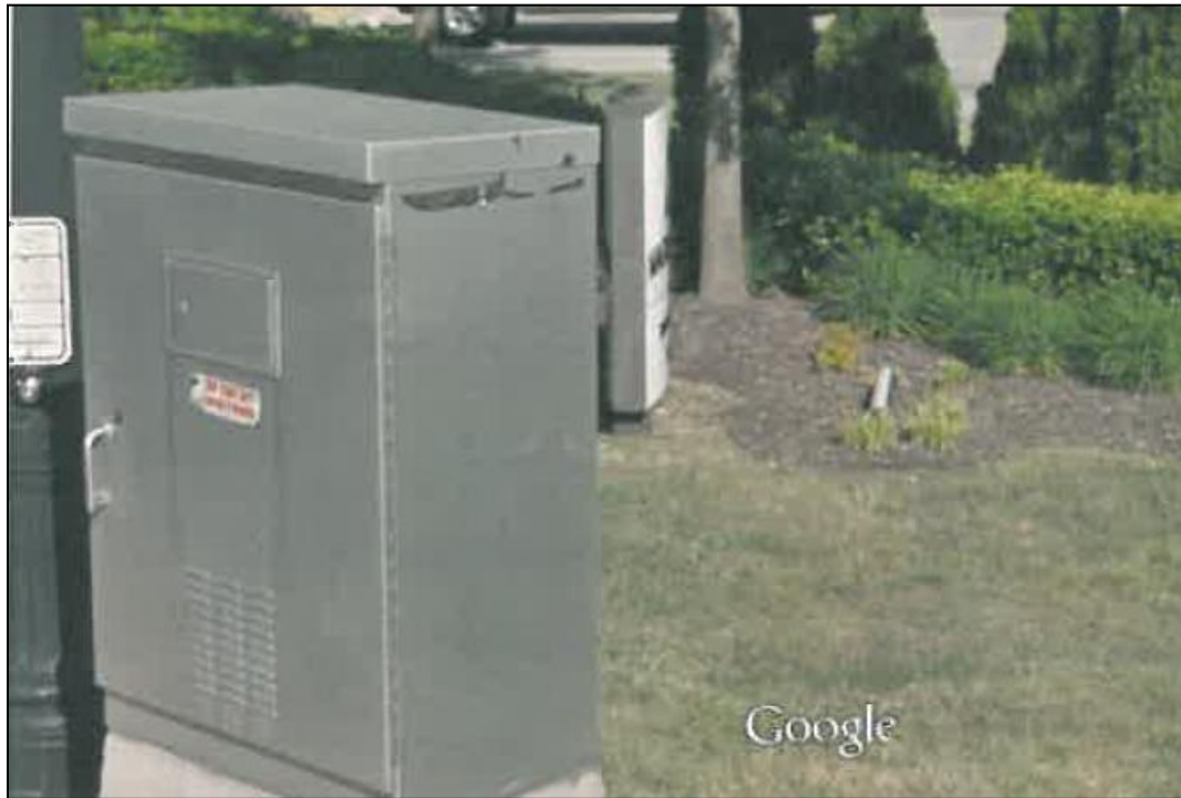
EXISTING GROUND LIGHTING
