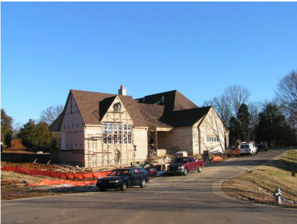
Side façade of home on Lot 1, as viewed from south (Dr. Martin Lane). The home is set back 10 feet from the roadway.
