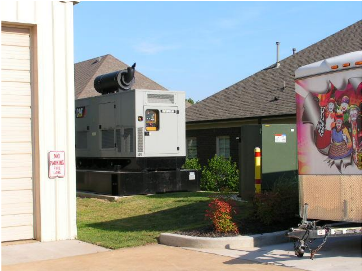
Looking northwest at the emergency generator and office building.
